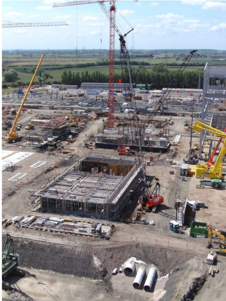
West Burton CCGT Power Station
