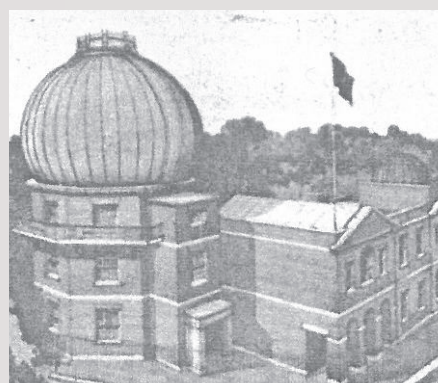
The tubular steel dome frame, weighing 12 tons, is lowered towards waiting workmen who will help in setting it into position atop the Great Equatorial Building.
